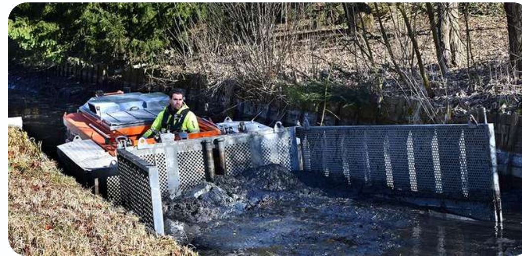
Floating Silt Pusher/Collector
